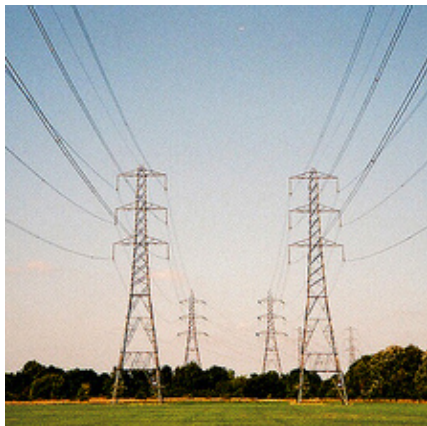
Electricity Pylons by Nick Page, on Flickr
